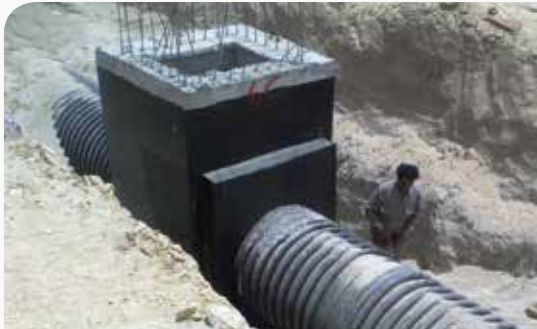
NIC HDPE Corrugated Pipes for Storm Water, connecting to Concrete Manholes at project in Kuwait
