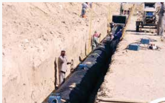
NIC HDPE Corrugated Pipes for Storm Water with electro-fusion connection at project in Kuwait
